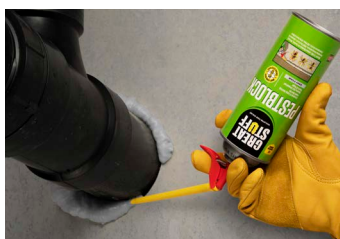
PVC Pipe Penetration
